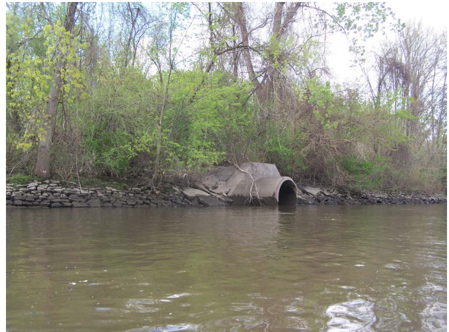
Sewer outfall along the Hudson River
